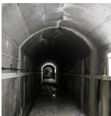
图 11 灌浆平洞钙化现象 Fig.11 Calcification in grouting adit
